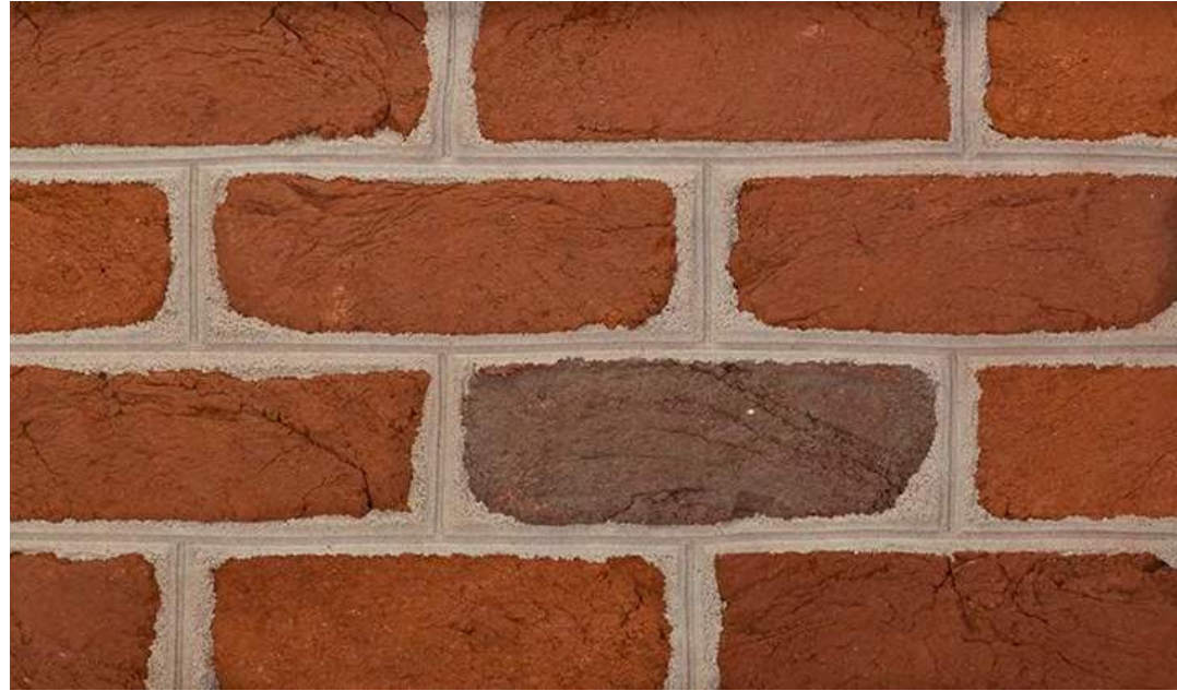
Hand Moulded Brick Infill at Damaged Areas of Existing Courthouse Glen-Gery - Virginia Blend Handmade
